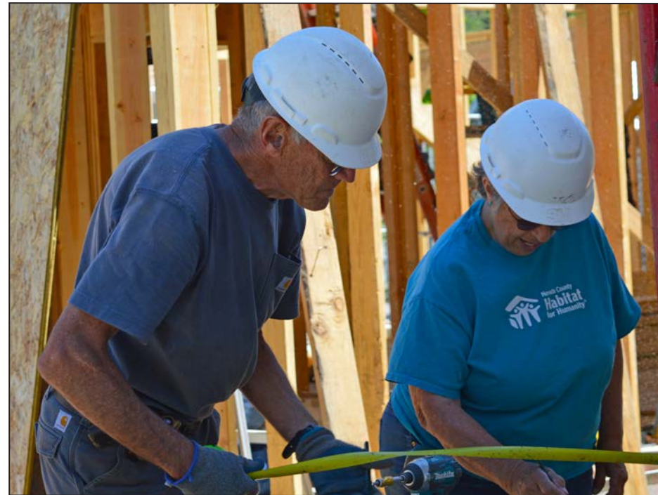
C.J. and a Habitat volunteer work together to build a house. Photo by Andy Wright.
